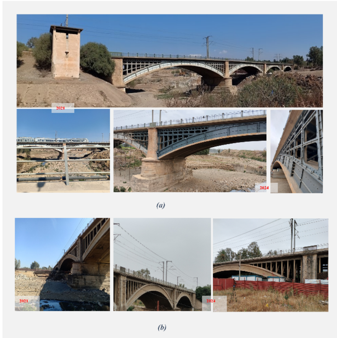
Fig. 1. Current state of cast-iron bridge (a), Current state of second reinforced concrete bridge (b)
