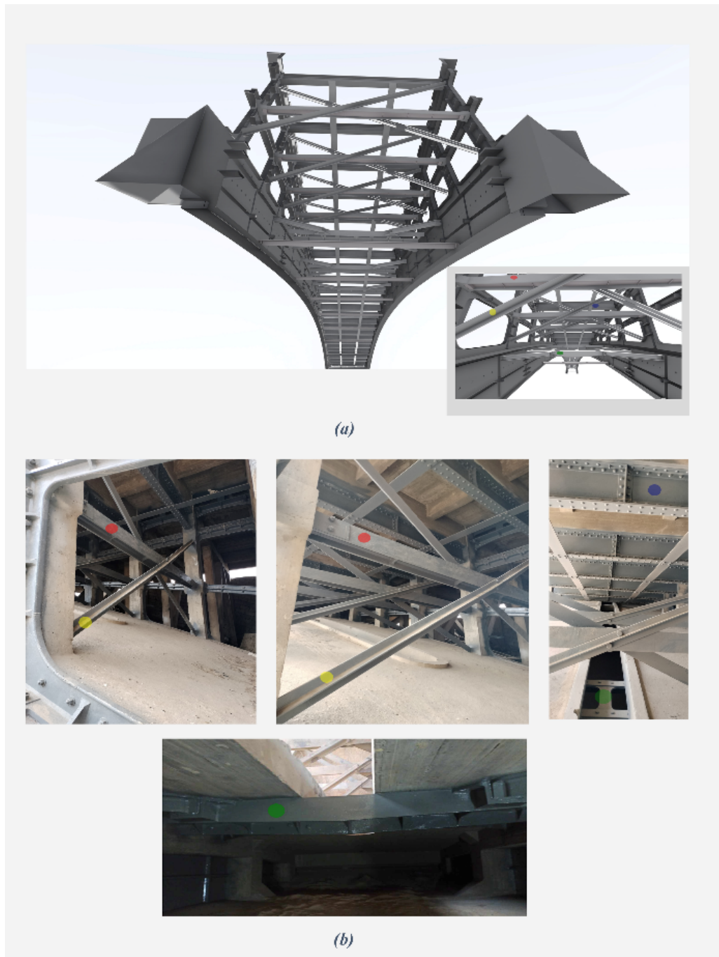
Fig. 4. Volumetric restoration tests of the state of the struts before reinforcement (a), Current state of the struts (Authors 2024) (b).
