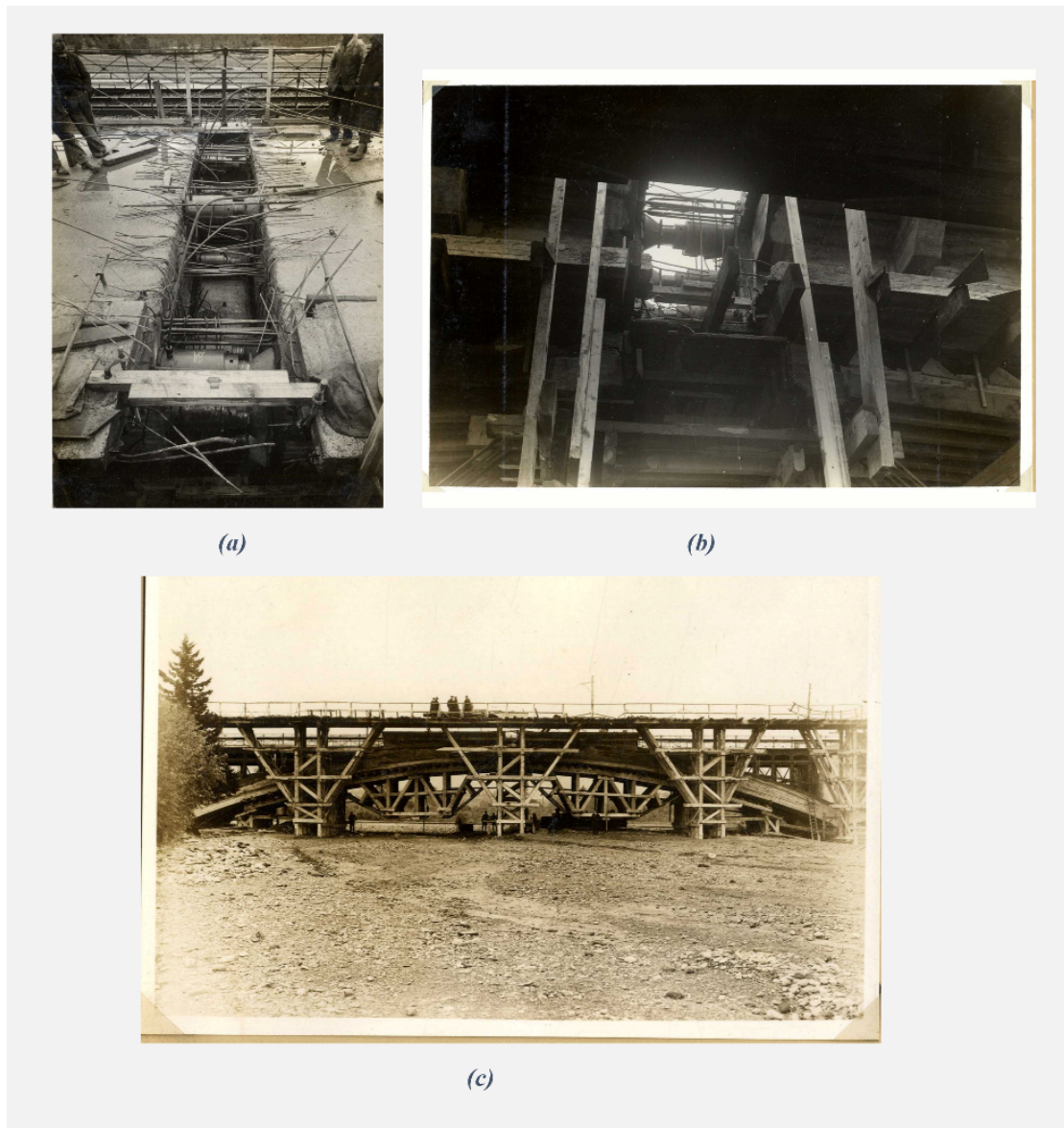
Fig. 10. Plan view of the key cut, and the rulers measuring horizontal displacements (a), view taken under the cast-iron bridge, showing the jacks in elevation in the key cut, in front of the ruler measuring vertical displacements (b), Wood shoring of the arch of the structure (c). (Established by Boussiron, “Décintrement des arcs pont sur l’oued Chiffa”, 1932, Box 169A, Hussein Dey.)
