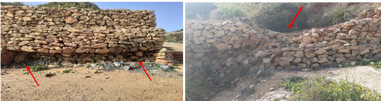
Photo 10 and 11: Cutting of the metal mesh leads to movement of stones and instability of the gabion threshold
