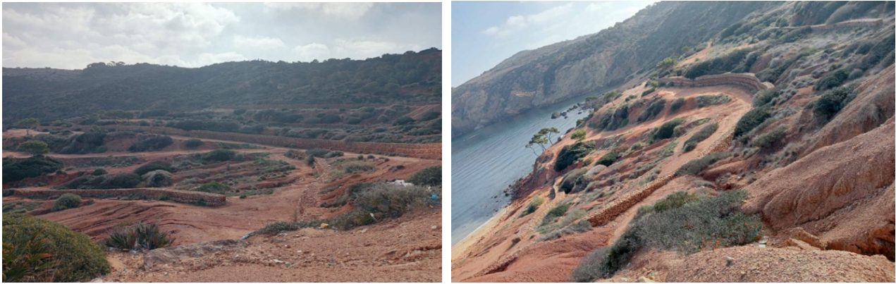
Photo 1 and 2: Station 1 of Sidi Driss beach protected against water erosion by gabions built in the form of walls
