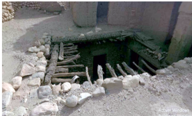
Photo no. 6: Disintegration of roof components due to head erosion. Source : Authors.2024.
