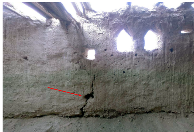
Photo 9: Punching crack caused by poor load distribution on the wall. Source : Authors.2024.
