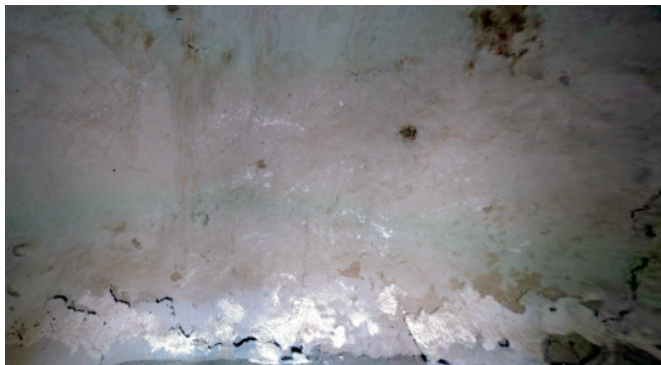
Photo 2 n°: Damage to the bottom of the wall caused by efflorescence, with detachment of the coating plaster.
