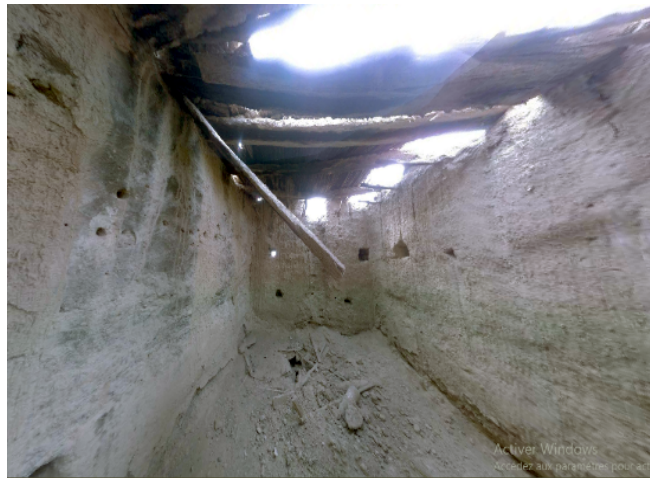
Photo 5: Damage caused by run-off, infiltration, internal condensation and wind. Source : Authors.2024.
