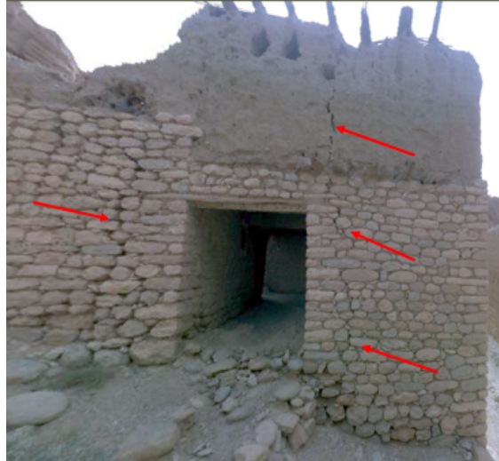
Photo no. 10: Differential settlement of foundations due to sloping ground and additional loads. Source : Authors.2024.
