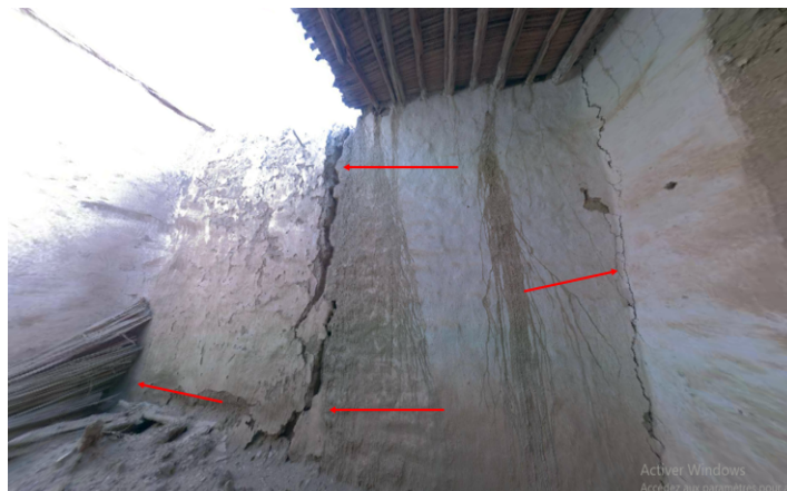
Photo 11: Damage caused by overloading, damp and wind. Source : Authors.2024
