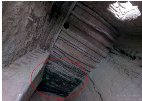
Photo n°4: Development of mould on juniper wood caused by condensation, infiltration and poor ventilation. Source : Authors.2024.
