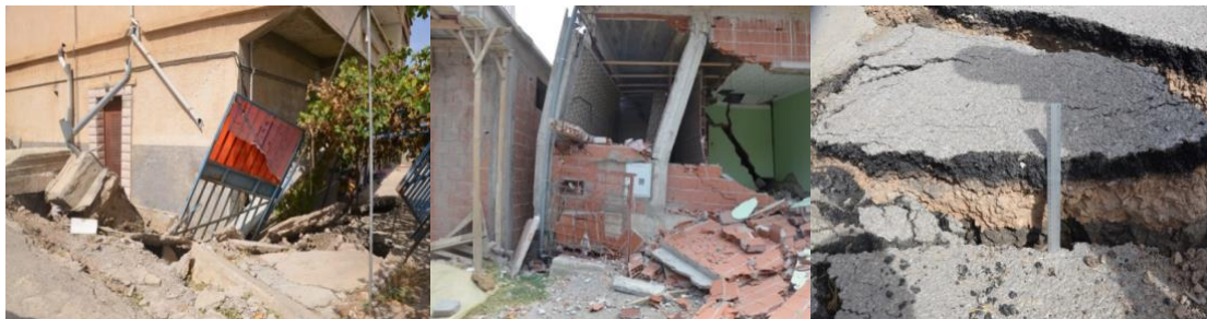
Figure 2. The damages in the kherba district The population is unaware of the importance of geotechnical studies and the necessity to build on soils compliant with current regulations. (source: author).
