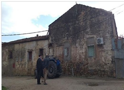
Figure 9. Farm in a state of disrepair Source: Authors, 2022.
