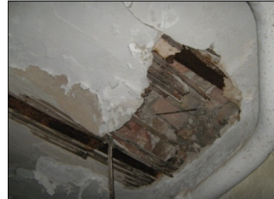
Cracks and detachment of the concrete in the new sanitary block.
