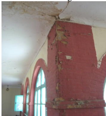
Detachment of roof cladding and solid brick due to dampness.
