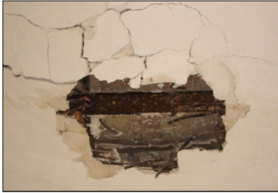
Cracks and detachment of the concrete under the stairwell leading to the upper floor.
