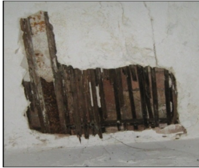
Deterioration of the roof in the the circulation area leading to the staircase.
